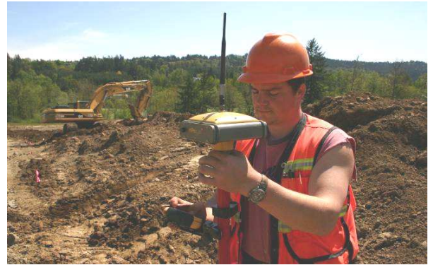
Matt Brockamp, Surveyor / Staker for NSP, staking curb & catch basins at Illahe Heights
